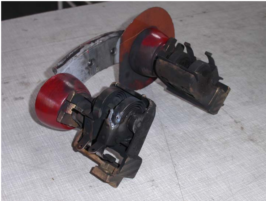
Fig. 8. The cracked and burned out brushholder's spring
