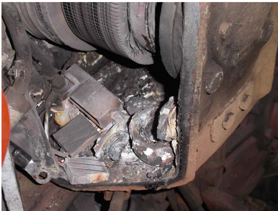
Fig. 7. The ruined brushholder and the damaged supplying cables
