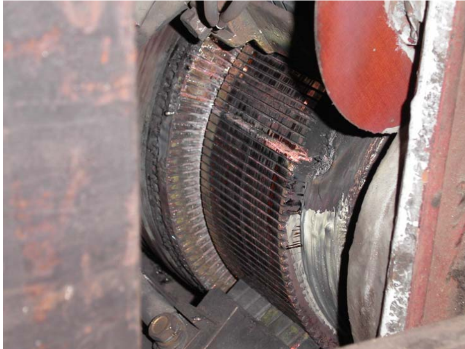
Fig. 6. Ruined commutator and the damaged shrouding
